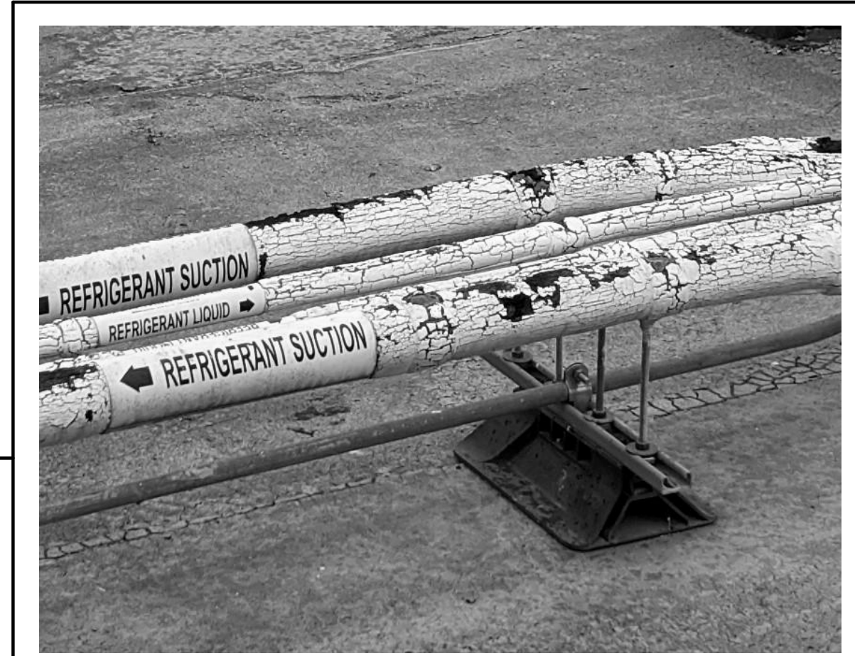
F REFRIGERANT MAINS, SYSTEM #4
