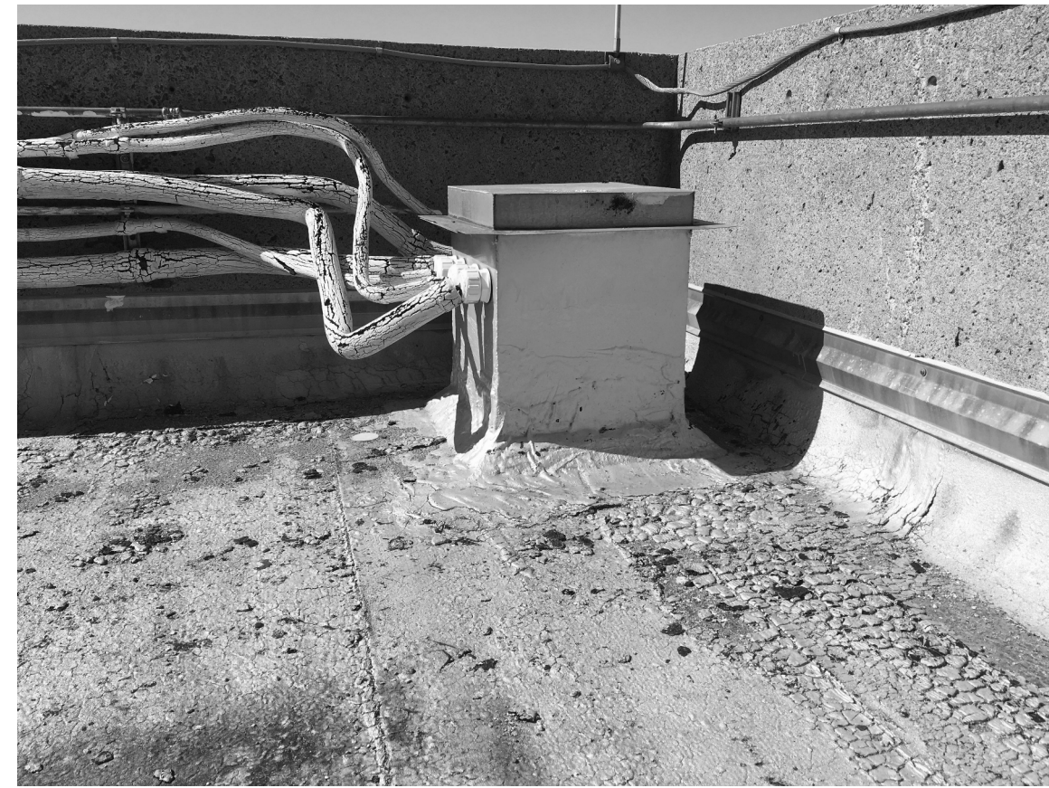
C REFRIGERANT PIPING AT ROOF CURB, SYSTEM #4
