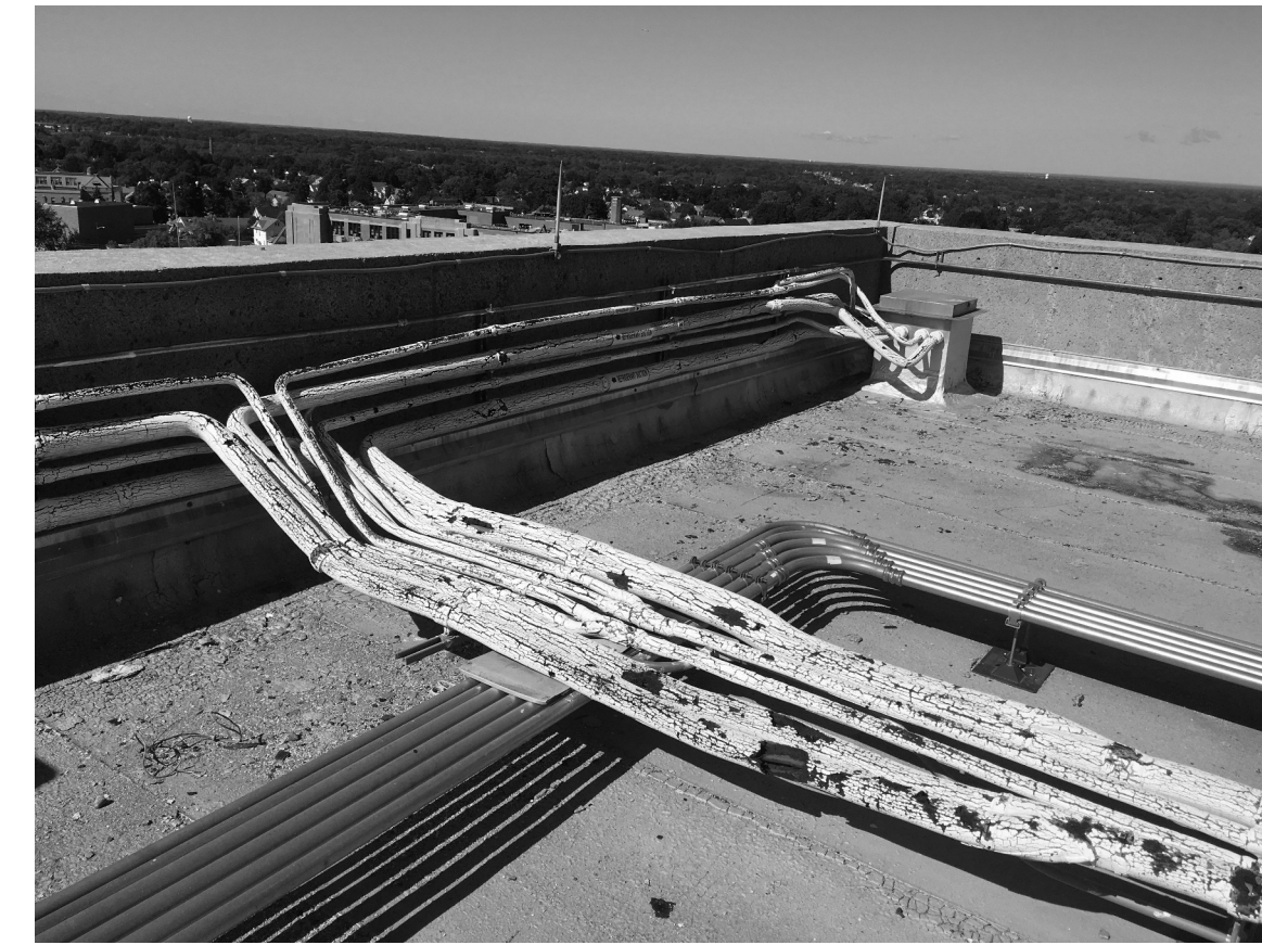
D REFRIGERANT PIPING AT MAINS, BRANCHES, WALL-SUPPORTS AND ROOF CURB, SYSTEM #4
