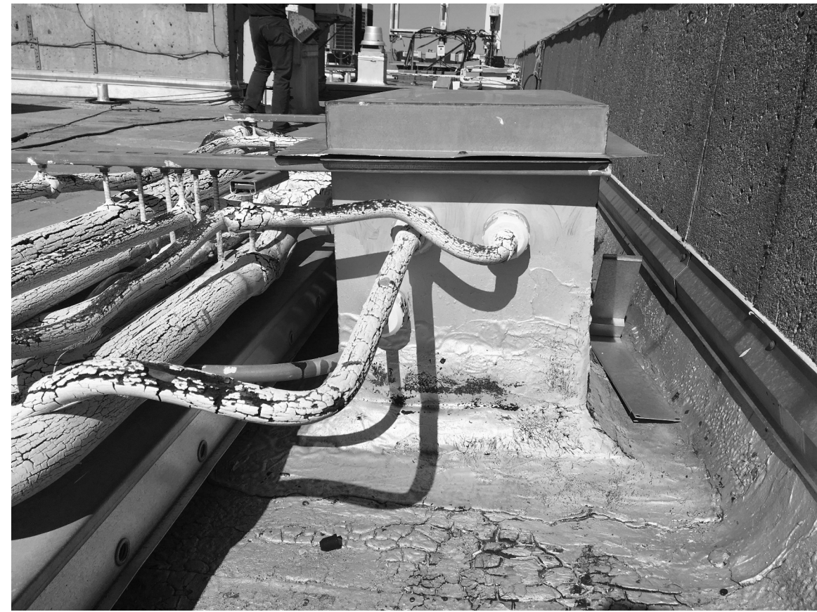
B REFRIGERANT PIPING AT ROOF CURB, SYSTEM #6
